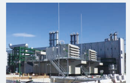
Gunma Complex (Gunma Prefecture), which is increasing its electricity self-sufficiency by adding gas turbines for power generation
