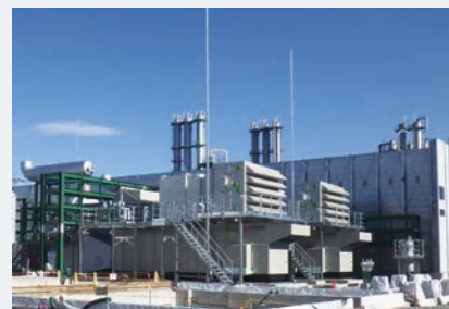
Gunma Complex (Gunma Prefecture), which is increasing its electricity self-sufficiency by adding gas turbines for power generation
