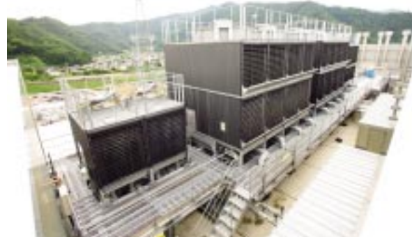
Cooling tower facilities
