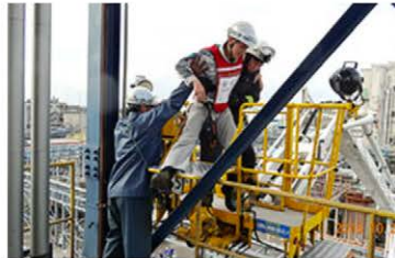
Drill for rescue of injured people from high places (October 2018, Shin-Etsu Chemical Naoetsu Plant)
