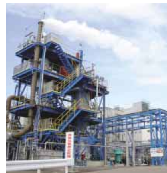
Combustion Facility (left front) and Recovery Facility (right bottom) of the Recycling System (What appears to be coming out from the stack is the steam.)
