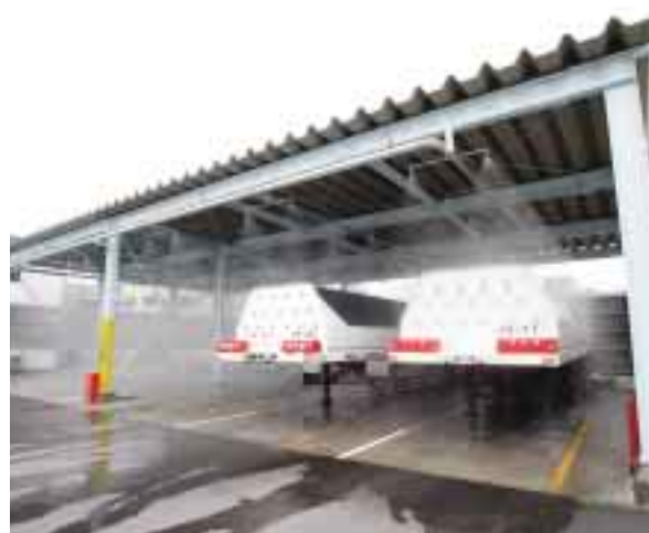
Water sprinkling firefighting test, based on the assumption of a hydrogen leak and fire
