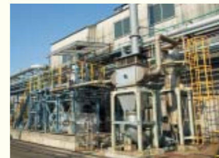
Off-gas and waste liquid incinerator
