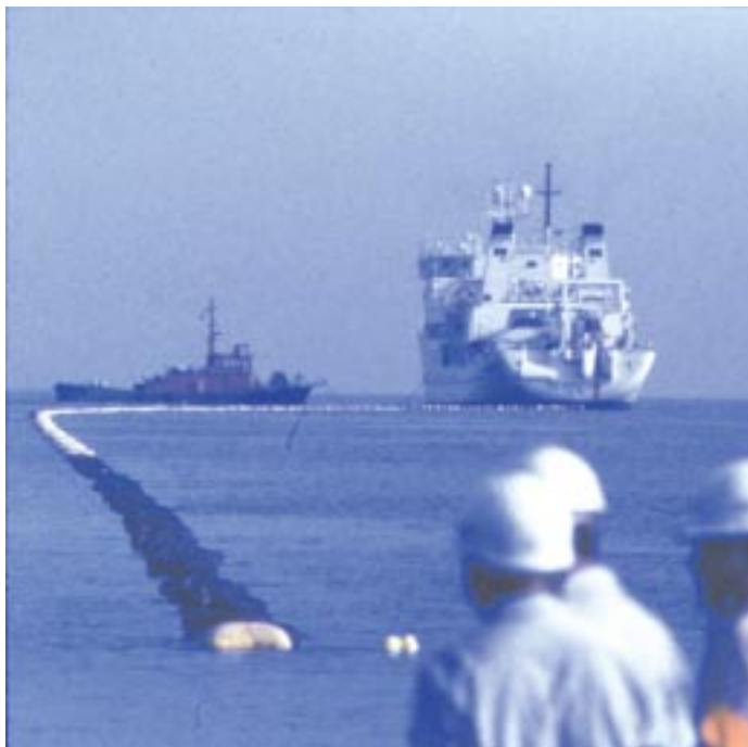
By expansion of undersea optical-fiber cable networks, global communication becomes ever easier
