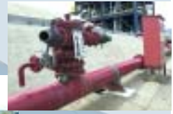
Hydrant for fire-truck use
