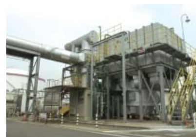
Waste emission treatment facility
