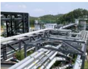
Wastewater treatment facilities
